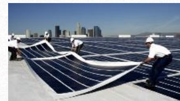
Solar Energy Cells on PVC Roofing Membrane
