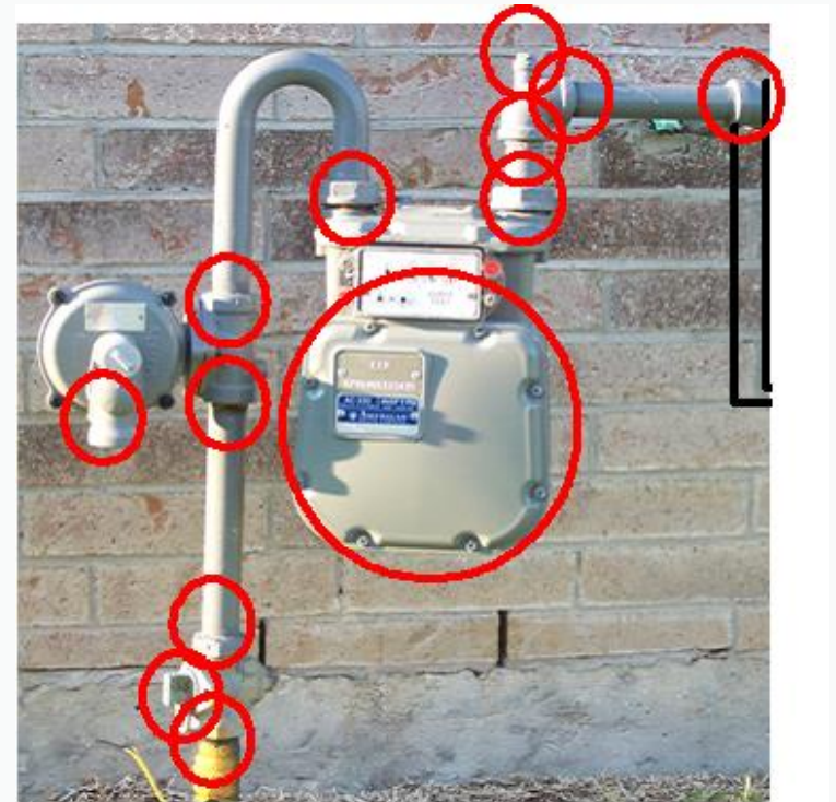
Gas Meter 13 Fugitive Sources
